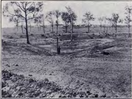
Council's Engineer standing in the foreground shows depth of filling which was necessary.
