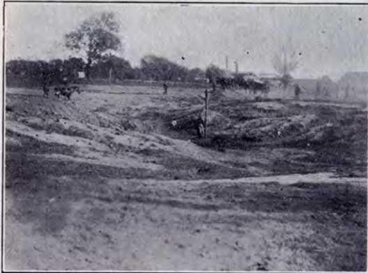
Site of present Oval, showing land that was reclaimed; (first week's work).
