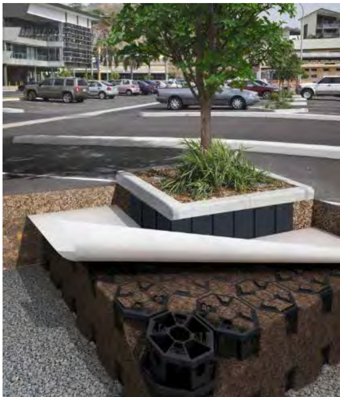
Example of using strata cells around hard surfaces (Photo courtesy of greenblue.com)
