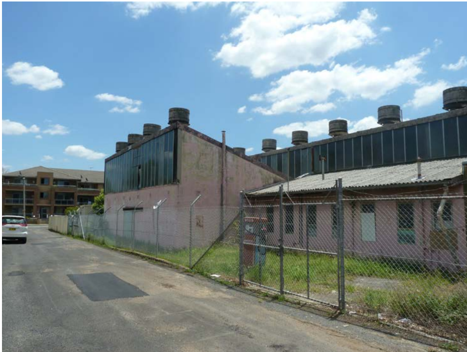
Figure 6 – Rear of the commercial warehouse building at 12 William Street, viewed from the access lane Source: JBA
