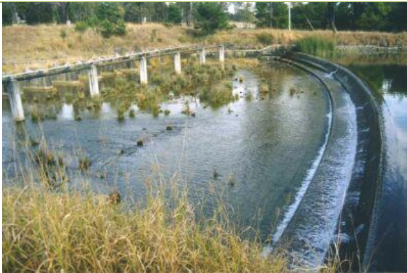
By-Wash Channel (Source: NSW Office of Environment and Heritage, State Heritage Register listing sheet for Prospect Reservoir)
