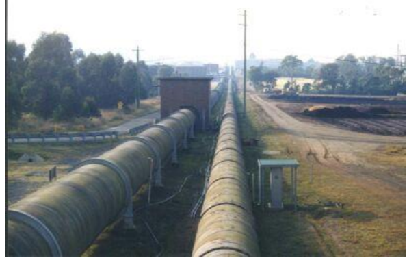
Pipelines (Source: NSW Office of Environment and Heritage, State Heritage Register listing sheet for Prospect Reservoir)
