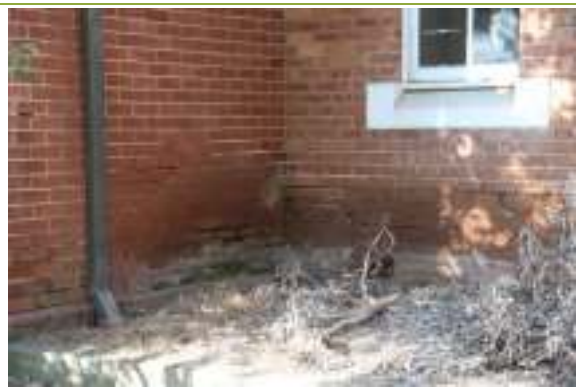
Detail of brickwork with severe salt attack on elevation to Arthur Street.
