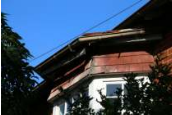
Detail of timber rot to shingles on bay window to Arcadia Street.
