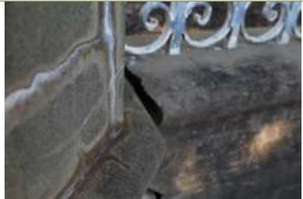
View of cracking due to ground settlement at the northern end of the Gates.
