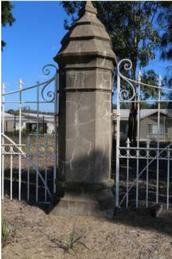
Cracking and efflorescence in the render.
