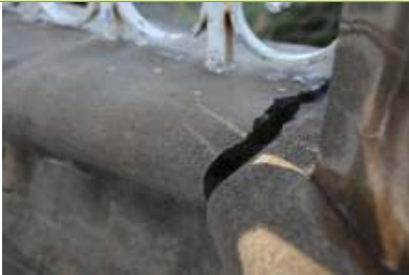
View of cracking due to ground settlement at the northern end of the Gates.
