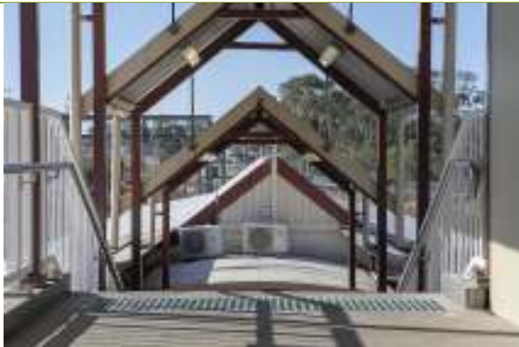
Platform canopy leading down to platform from footbridge (Source: NSW Office of Environment and Heritage, Railcorp S170 Listing Sheet for Regents Park Railway Station Group).
